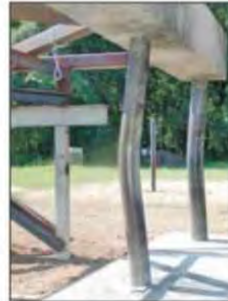
Buckled Steel Column
