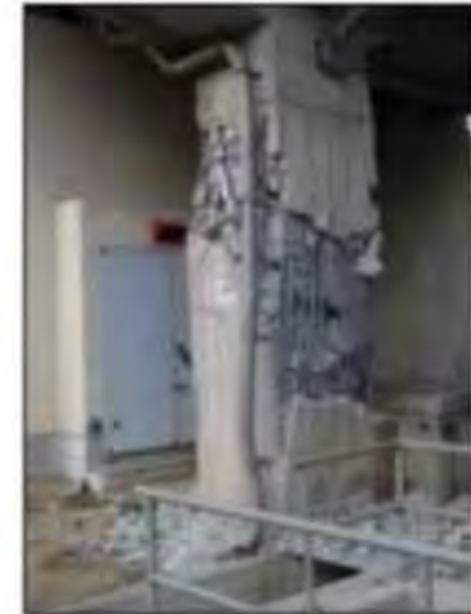
Buckled R.C.C. Column
